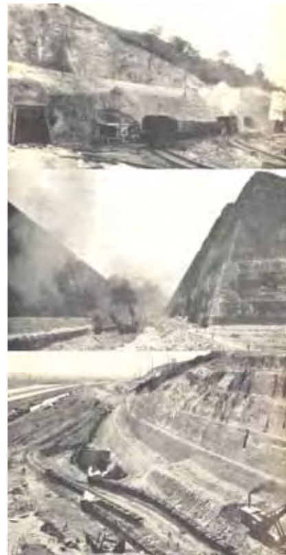
Figure 13. On top: The entry to the muck tunnels in the Sint Pietersberg. These were constructed and used only during the excavation of the Caster trench. In the middle: Steam shovels at work in the Caster trench. Below: Muck trains in the Caster trench on the level of the canal, in the distance: the river Maas (Photos modified after Delmer 1939).
