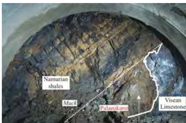
Figure 15. Tunnel front during the construction of the Soumagne tunnel (radius 5.5m) showing the Palaeokarst on the Namurian-Visean interface (Photo: Courtesy of S.M. Soumagne Tunnel).
