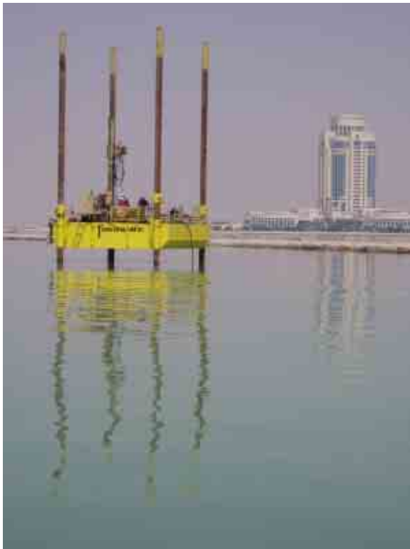
Figure 1: Fugro's nearshore jack-up rig Geo Giant drilling for Pearl of the Gulf Island, Doha.
